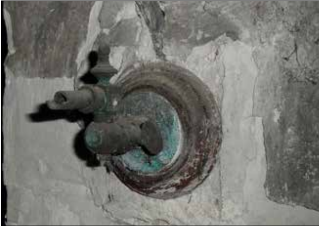
An example of an original gas fitting and connecting pipe
