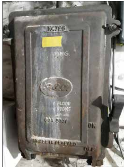
An early 1930s electrical box
