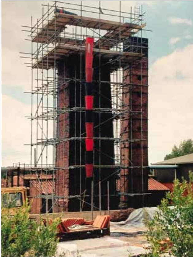
Fig. 1 The beheading of the Hoe Hill Hoffmann chimney in progress in 2018. Fortunately, the complete destruction of this Grade II Listed Structure was prevented just in time. To its right can be seen the more slender chimney now used during the firing of the yard's two remaining down-draught kilns. (Geoff Bryant)
